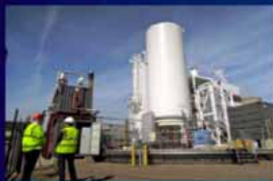
Liquid Air Storage TRL 7
