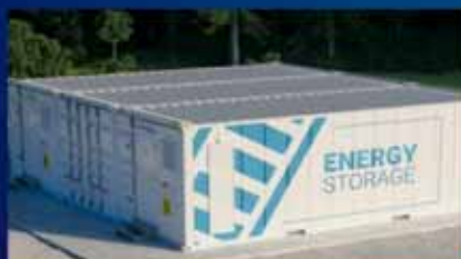
Grid Scale Batteries TRL9
