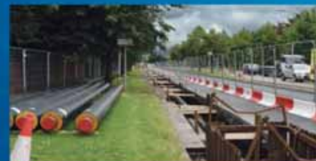
District Heating (4G & 5G) TRL 8-9
